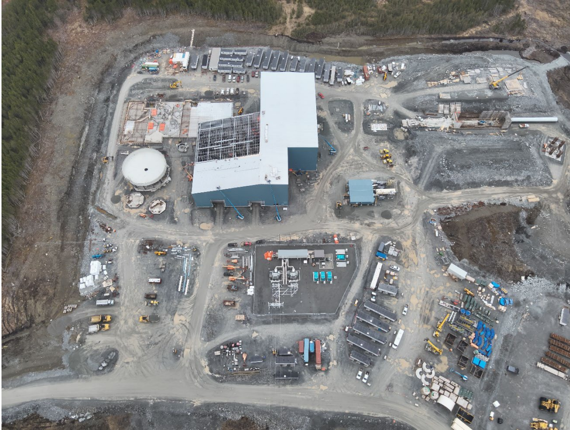
Process Plant East
